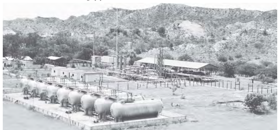
Lequified Petroleum Gas Plant (Kyunchaung).
