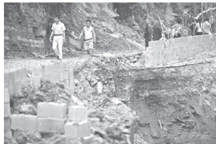
People walk on the road destroyed in heavy rainfall in Daozhen County of Zunyi City, southwest China's Guizhou Province, on 11 July, 2010. About 153,900 residents in the county have suffered a lot from the heavy rainfall which lasted for three days from 8 July.
