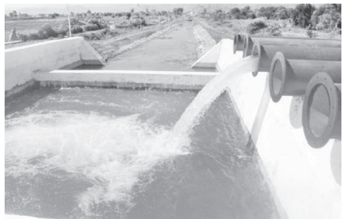
Dahseik River Water Pumping Station in Dahseik Village, Langkho Township, Shan State (South).
