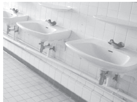
Thieves have robbed a newly renovated police station in South Africa, stealing everything down to the kitchen sink.
