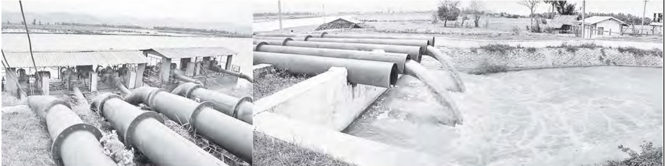
The intake structure of Shanywa River Water Pumping Station on the bank of the river Paunglaung.
