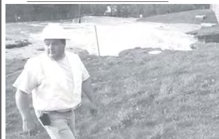
Water surges from the ground at the site of a water main break, on 1 May, Saturday, 2010, in Weston, Mass. Water to 2 million people in Boston and more than two dozen suburbs is temporarily unsuitable for drinking after the break in a pipe that connects a major suburban reservoir to the city.—INTERNET
