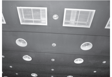
Advanced sound system installed at Aung Thabye modern cinema.
