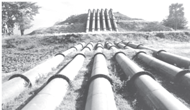
The 30-inch diameter pipe to pump water.
