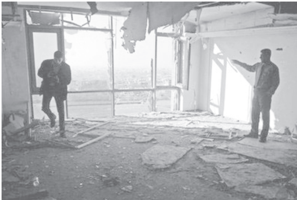
People inspect a rocket attack damage to the new U.S. consulate building in Herat, west of Kabul, Afghanistan, on Saturday, 9 Jan. 2010.
