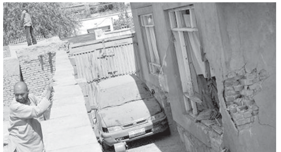
A man checks the remains of a damaged house which was hit by a rocket Sunday night, killing three family members while sleeping in their house in Kabul, Afghanistan recently. —XINHUA
