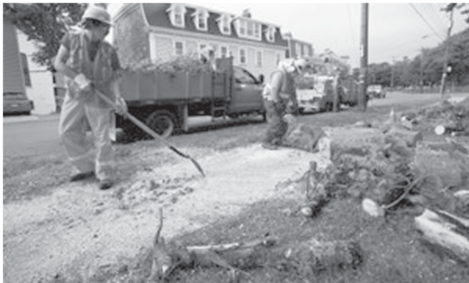
St John’s municipal workers clean up following Tropical Storm Bill which blew into St John’s early on 24 Aug, 2009. There were only minor damages from the high winds as Bill quickly passed over the Avalon Peninsula.—INTERNET
