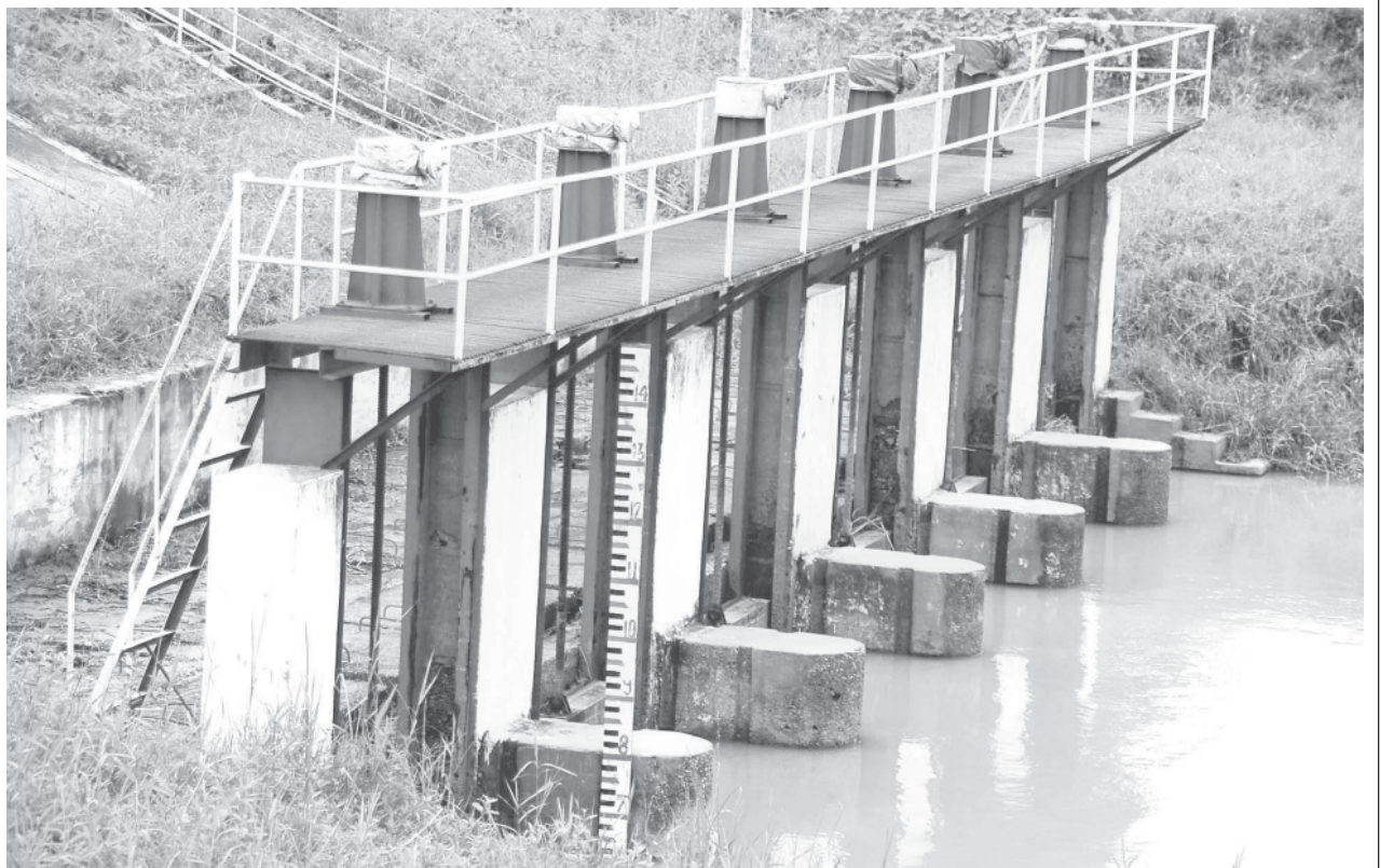
The gates of Wadaw Sluice Gate.
