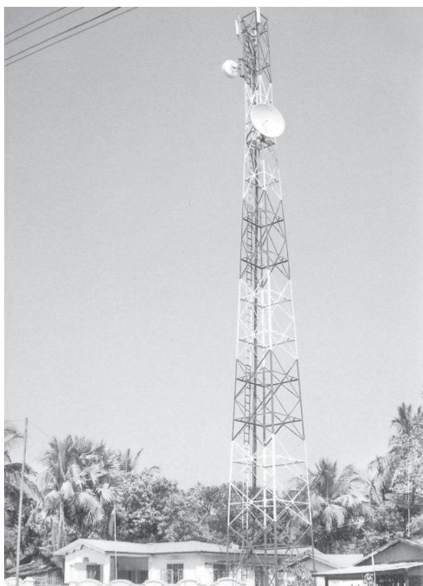
Phayagyi Village microwave station on Yangon-Mandalay Union Highway in Bago Township.
