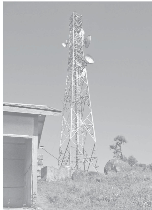
Photo shows a microwave station in Mongpyin.
