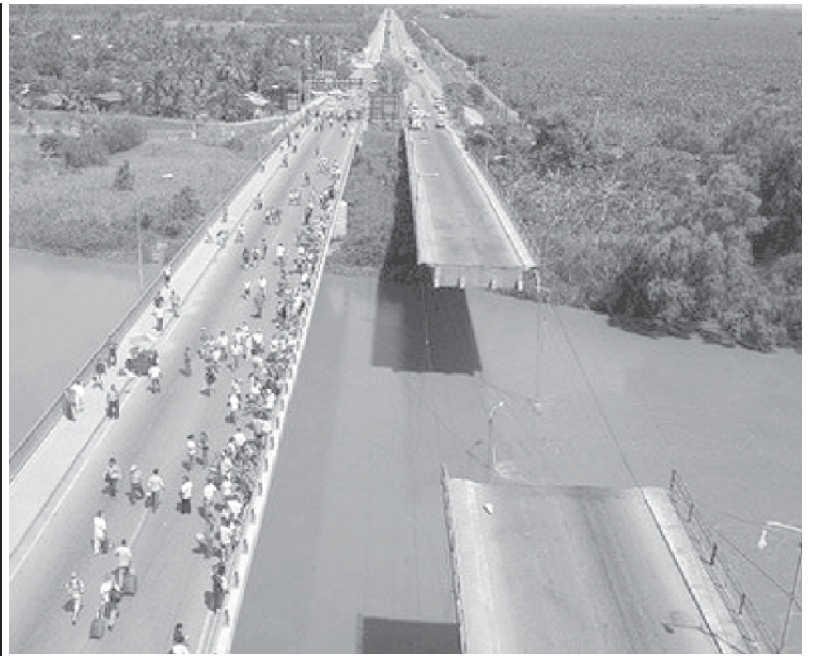
One of the lanes of ‘La Democracia’ bridge over the Ulua river, built by the French in 1963, had its central section collapse due to an earthquake in El Progreso, 270 km north of Tegucigalpa. A powerful 7.1-magnitude earthquake rocked the economic and tourist heart of Honduras, killing five, wounding at least 13, and shaking neighboring countries as far away as Mexico.—INTERNET
