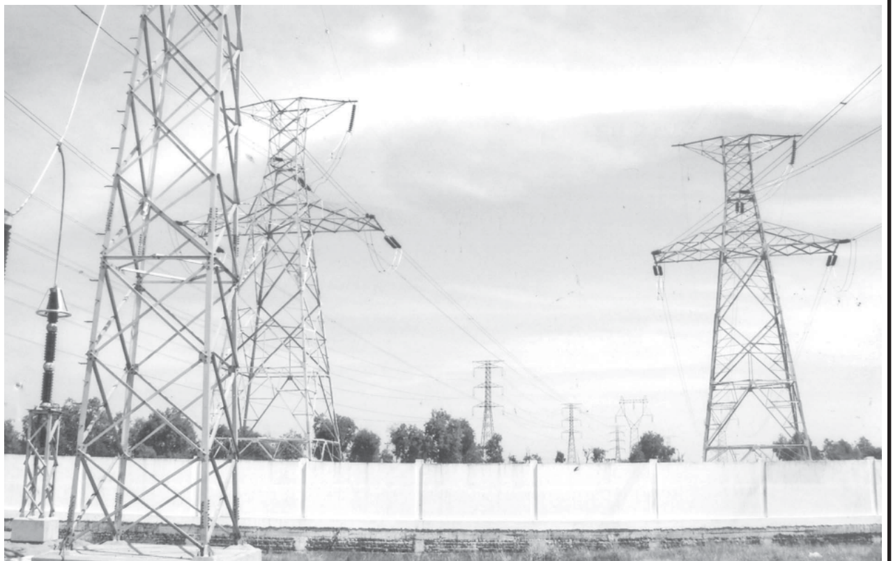
Kamanut-Myaungdaga 230 KV grid.
