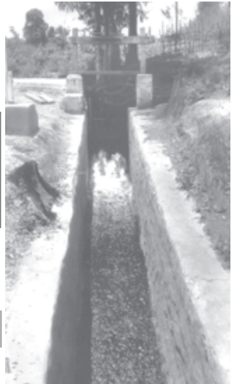
Water intake facility of power station that generates 15 kilowatts of electricity in Kehsi Township, Shan State (South).— PBANRDA
