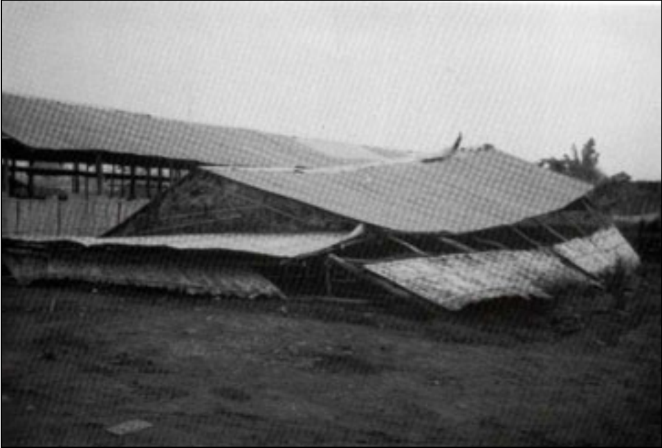
Photo shows the collapsed school building (above), where one of the students was killed (below). (Photo by KHRG)
