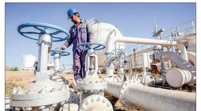
A file picture shows Iraqi oil employee checking pipelines at the Bai Hassan oil field, west of the multi-ethnic northern Iraqi city of Kirkuk. PHOTO: AFP/FILE
