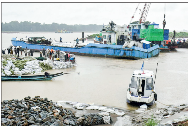
Recovery efforts are underway along the damaged section of the Ngawun River embankment.
