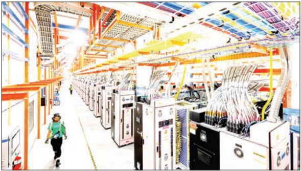
This image shows an AWS data centre facility in Indiana featuring pink server racks labeled “Project Rainier”. PHOTO: AMAZON
