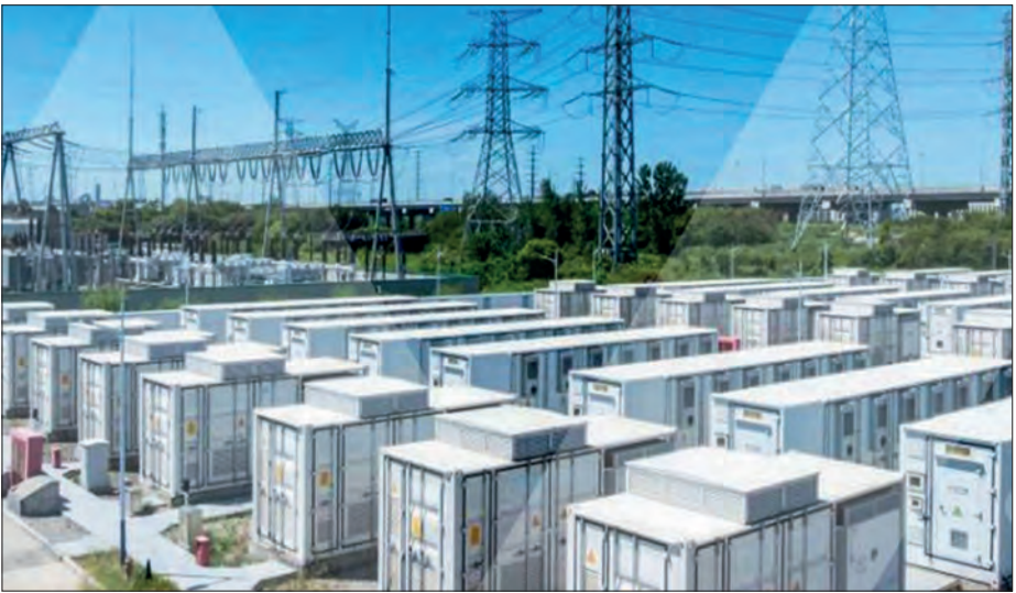
The image shows a large-scale, utility-grade Battery Energy Storage System (BESS) integrated with an electrical substation grid. PHOTO: ANI
