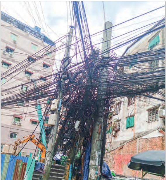
Disordered installation of telecommunication cables at a power pole in Yangon's Sangyoung Township.
