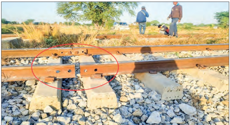
The complete destruction of the track plates, bolts and track clips at milepost 327/12-11 between Samon and Thaeday stations in Wundwin Township.
