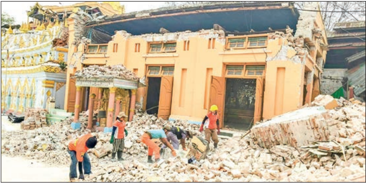
This photo captures some damage caused by the Mandalay earthquake.
