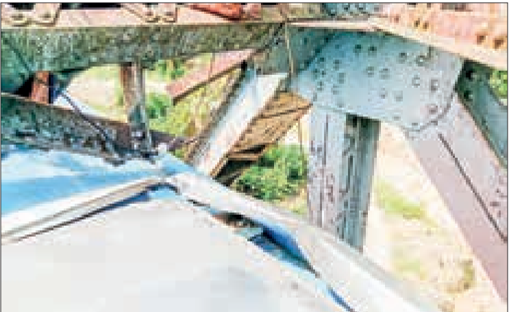
This image shows the fallen beam of Kabaung Bridge near Toungoo Railway Station.
