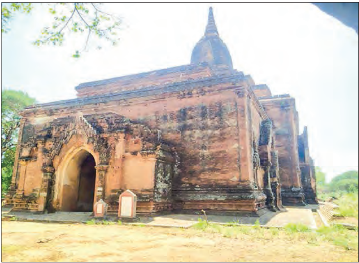
The crack caused by the earthquake in 2016 seen at Meenyeingon Temple in Bagan.
