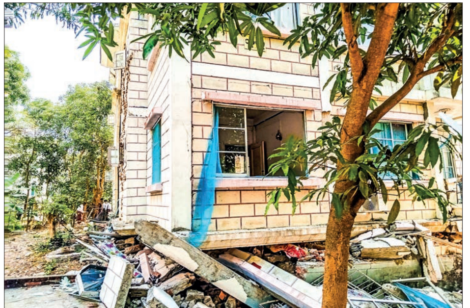
This photo shows the severely collapsed building No 1307 in Nay Pyi Taw.
