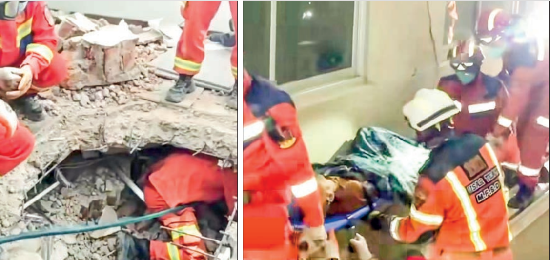
A rescue team from Yunnan Province of China evacuate a survivor trapped under the collapsed floor at Ottarathiri Hospital in Nay Pyi Taw on the night of 29 March.
