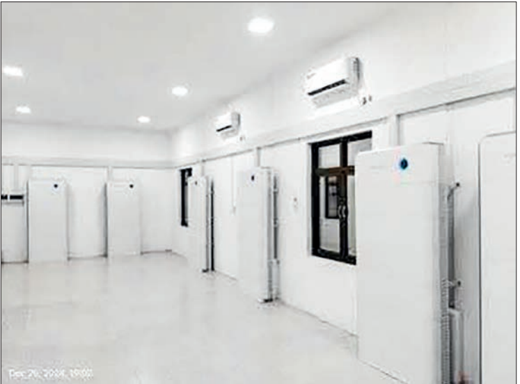
This photo shows solar power generation being implemented at the natural gas distribution station in Yenangyoung. PHOTO-SEAOP-SEAGP
