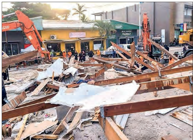
Australian rescue workers comb through the site of a collapsed building in Port Vila, the capital city of Vanuatu / © AUSTRALIAN DEPARTMENT OF FOREIGN AFFAIRS AND TRADE/AFP
