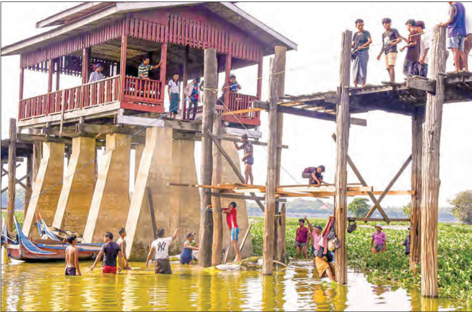
The damaged section seen under restoration.
