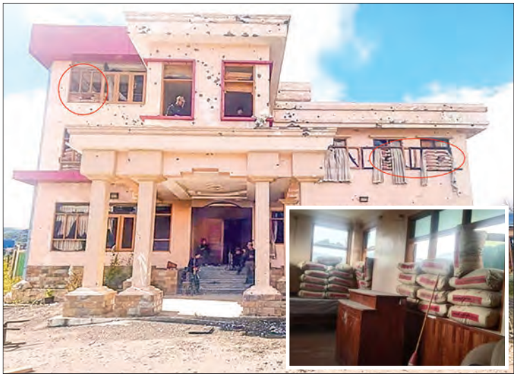
CNF and CDF terrorists use the public construction office building as bunkers and fortifications in Thantlang.
