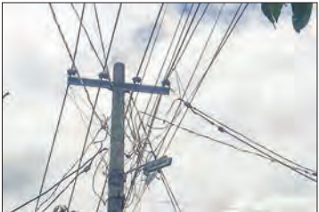
Electric cables connected to the lamp-post.
