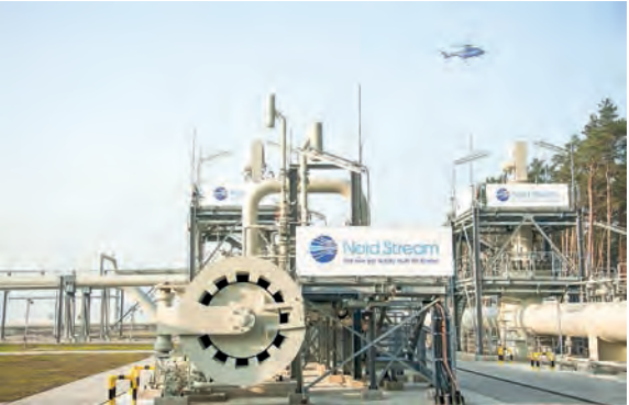
A helicopter flies over the Nordstream gas pipeline terminal prior to an inaugural ceremony for the first of Nord Stream’s twin 1,224 kilometre gas pipeline through the Baltic Sea, in Lubmin, Germany. 8 November 2011. PHOTO: AFP
