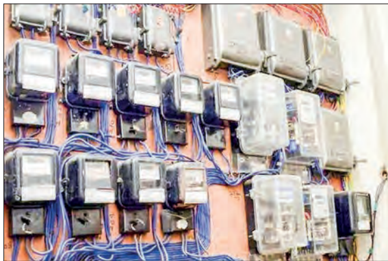
Meter boxes are seen at an apartment.
