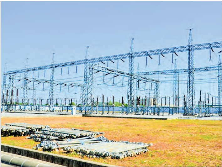
A power distribution sub-station.
