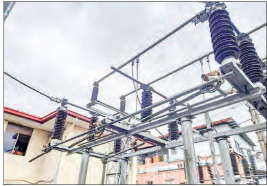
One power distribution station.
