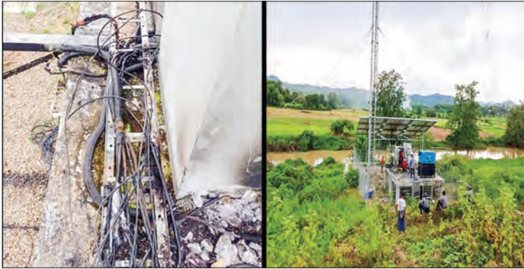
Mytel tower in Kanma Township.
