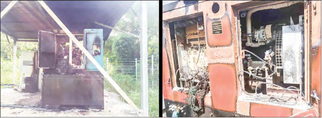
Two Mytel towers were destroyed in Kyantgin Township.
