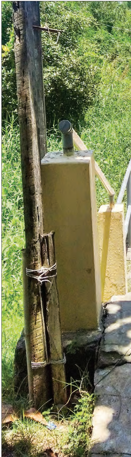
A bridge destroyed by erosion being seen.
