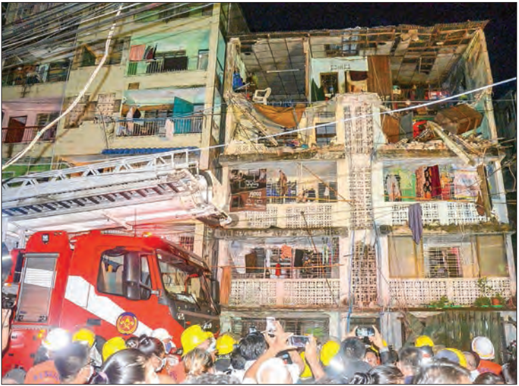
The collapsed veranda of the five-storey apartment seen in Sangyaung Township, Yangon. PHOTO: ZAW GYI
