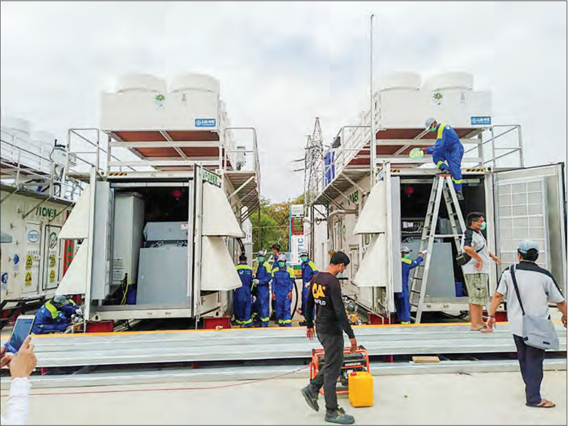
Electrical technicians seen at the Kyunchaung natural gas power plant in Magway Region . PHOTO: KO ZAW (CHEMISTRY)
