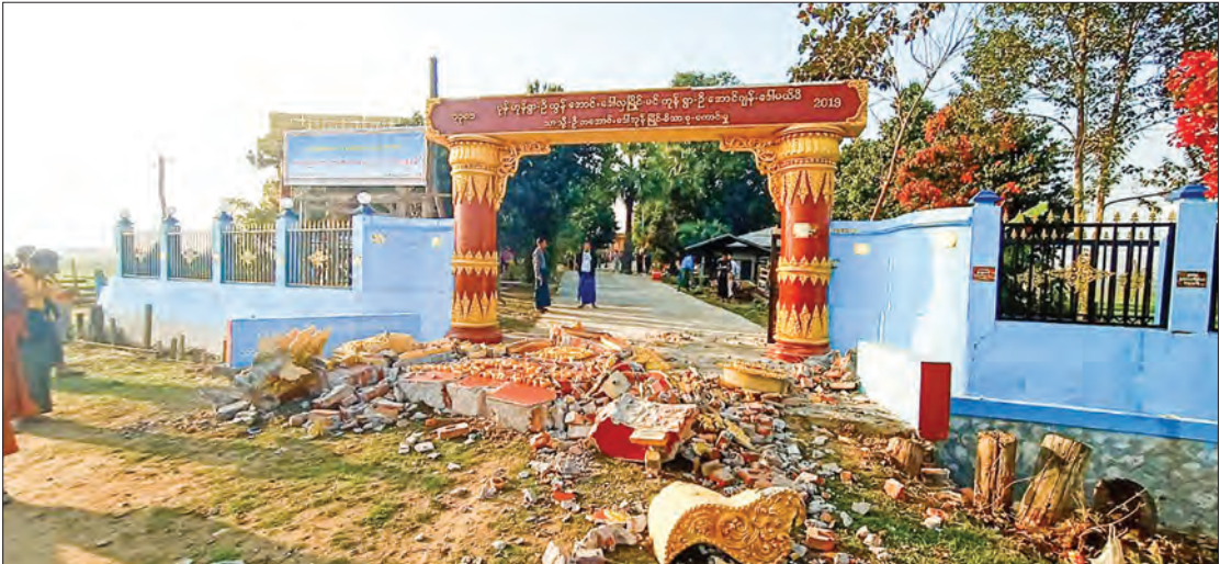
The collapsed bricks of the entrance gate of the Phone Kone monastery seen after an earthquake jolted Pone Hone village-tract in Indaw Township yesterday. PHOTO: MAUNG CHIT LIN (INDAW)
