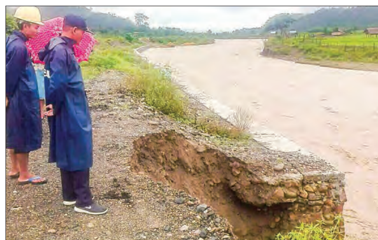
Flood in Moehnyin Township causes retaining wall collapse. PHOTO: NI TOE
