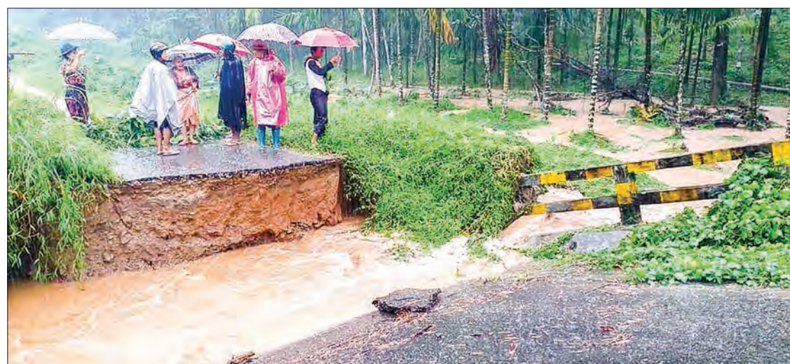
A bridge is destroyed by the flood in Kyunsu Township. PHOTO: SI THURA AUNG (KYUNSU)
