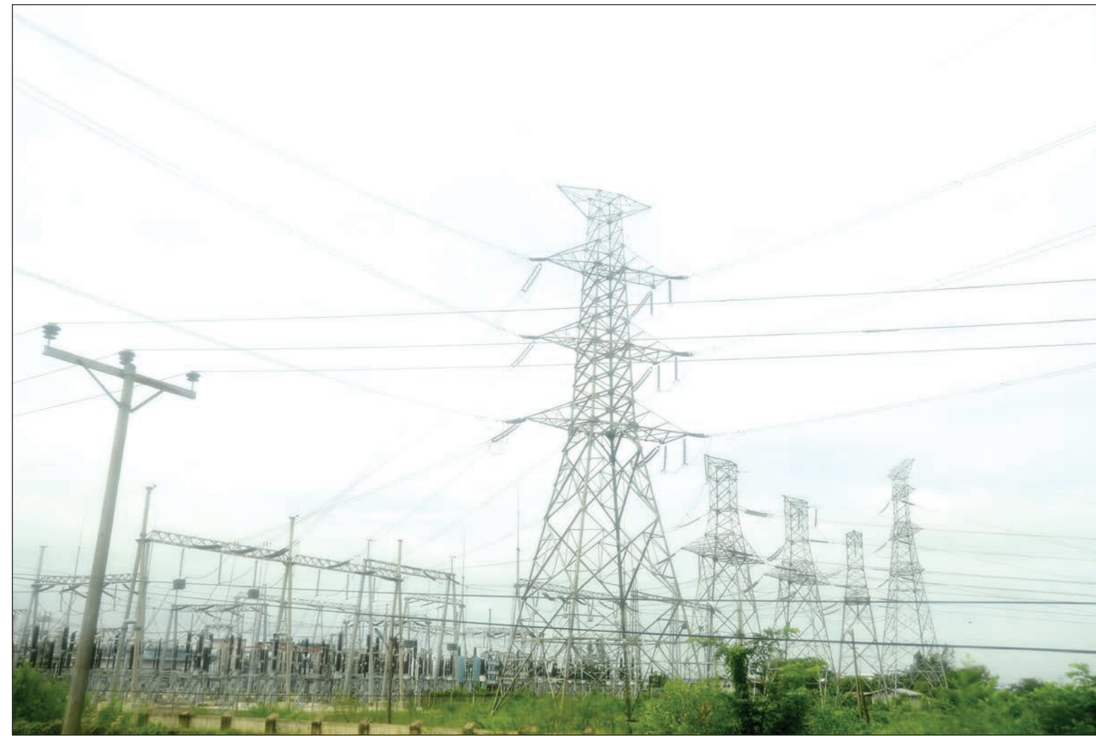
An electricity substation. PHOTO: PHOE KHWAH
