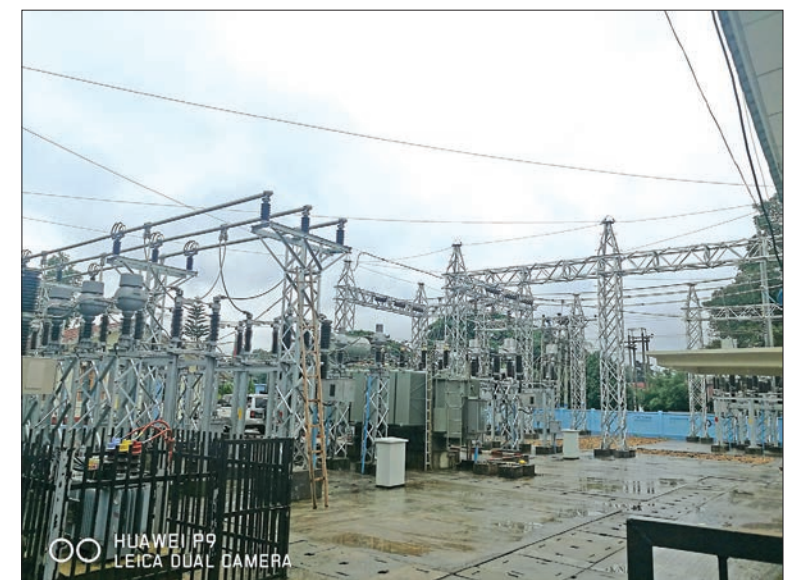
66 kV Mawlamyine-Thanyuayay Substation
