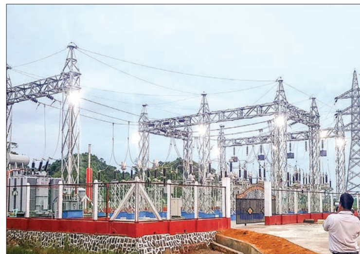
Buthidaung electrical sub-station in Rakhine State. PHOTO: MNA
