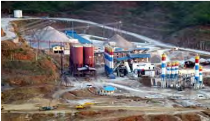
RCC & CVC Batching Plants
