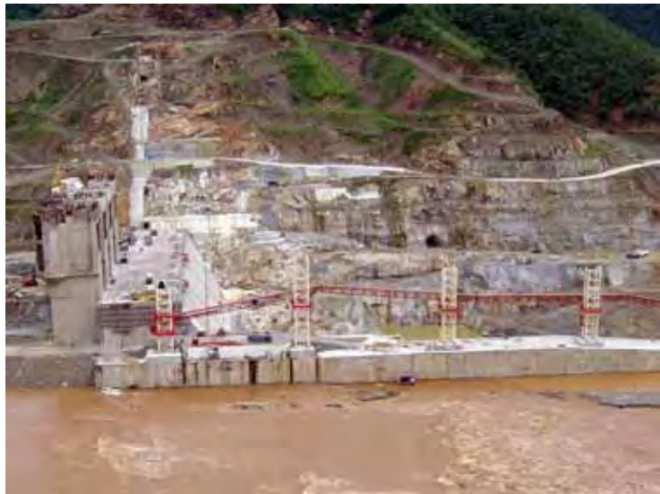
View from left bank shortly after major flooding Oct 06
