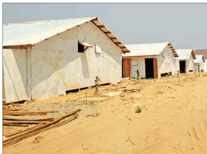
The construction of Hla Phoe Khaung Transit Centre expected to be completed on 31 March 2018. PHOTO: MNA
