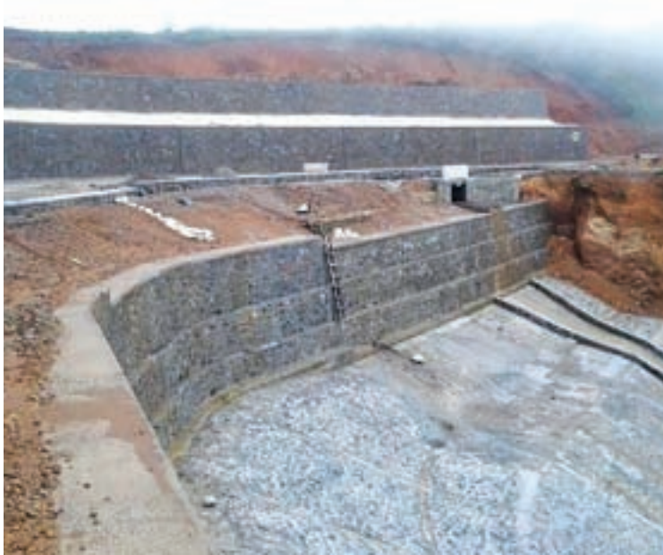
Retaining wall along the Minbu-An-Sittway Road. PHOTO: MNA
