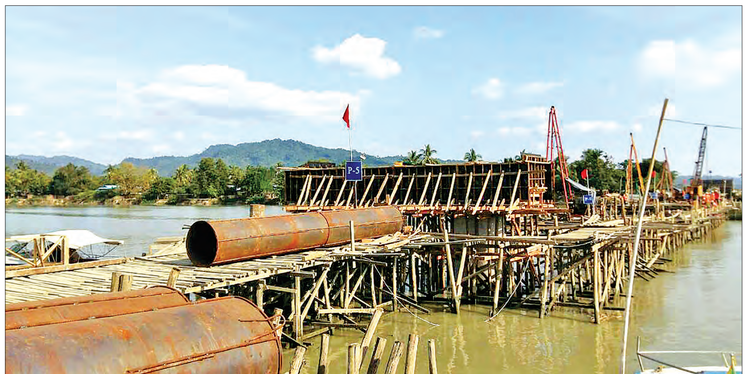
Photo shows the construction of 49-mile long Sittway-Maungtaw Road supporting Maungtaw region development, Rakhine State.
